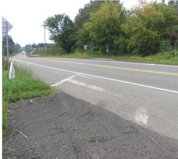
Figure 17. Crosswalk not repainted after road repaving, Pat McGee Trail, Little Valley, NY
