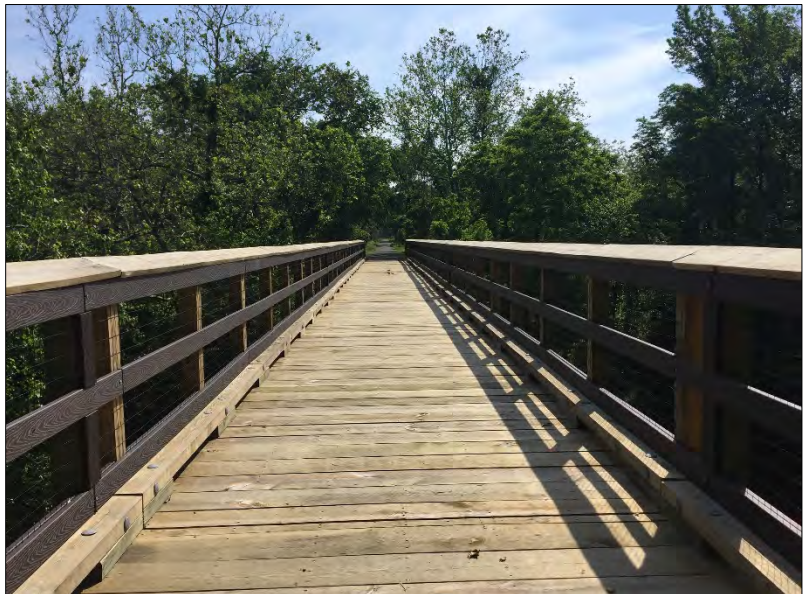
Image 24. Tuckahoe Railroad Bridge over Tuckahoe Creek - View looking east towards Tuckahoe State Park Rail-Trail. Credit: MD DNR.
