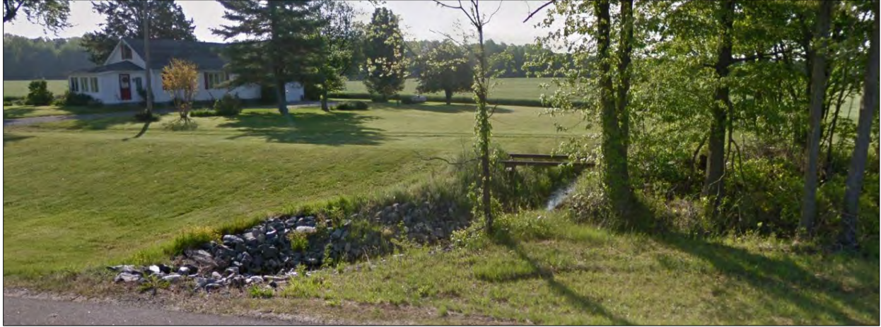
Image 15. Rail corridor tracks crossing over culvert drainage with no support underneath - View looking east, north of intersection with Klondike Road. Credit: GoogleMaps.
